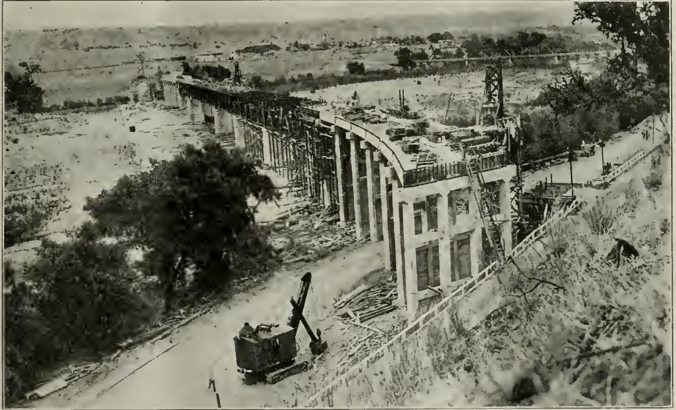
Bradley Bridge Over the Salinas River, Showing the Concrete Piers on Curve. A $265,000 Structure for the California State Highway Commission. Old Bridge Can be Seen at Right. New Structure to be Opened to Traffic Next Month. Lord and Bishop, Contractors.
